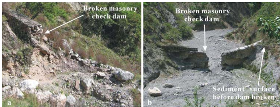
Fig. 5 Site photographs showing two broken check-dams in upstream of Duozhao ravine. a Broken check-dam in Xiaoya channel, position (3,140E–380N), by the impact of dolomite blocks from
